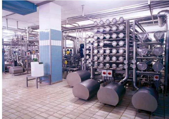
Fig. 12.6 Integrated membrane filtration system comprising UF plant for WPC & RO plant for lactose concentration
